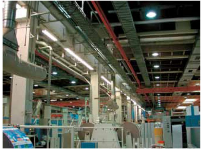
Cost-effective lighting is important in all production facilities, where ceilings are high and it is expensive to stop production. That is why Tetra Pak Produktions GmbH in Berlin use Aura Long Life lamps.
